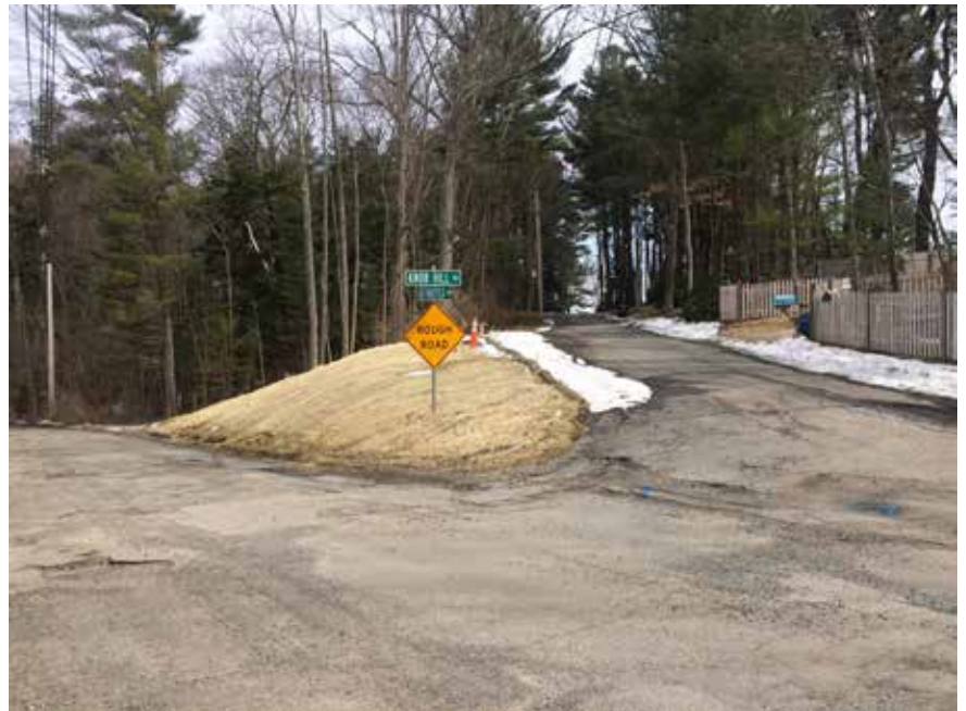
Improvements at Knob Hill are underway, when complete an enormous source of erosion-causing, unfiltered run-off will be eliminated.
